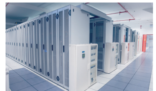
Project Mustang Due Diligence (Amazon Data Centers) - KSA
