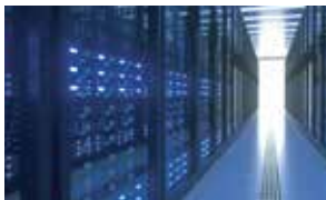
Data Center Site Capacity Assessment - KSA
