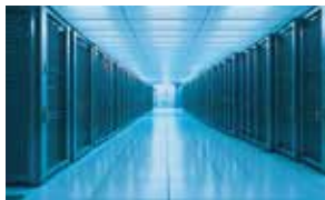
Mobily Modular Data Center - KSA
